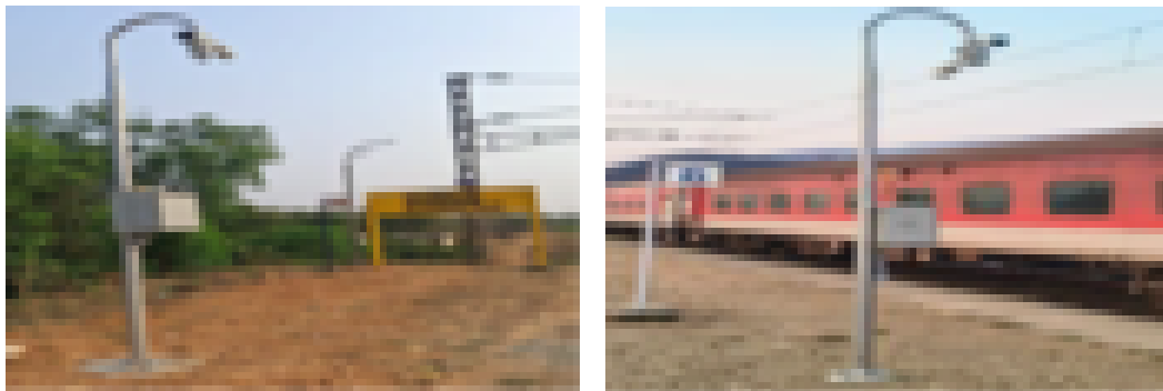
(CCTV camera installed at Achirne station)
