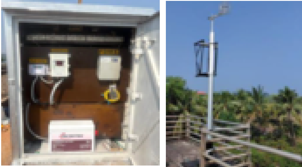
(Site Unit and Wind Speed Sensor installed at Sharavathi Bridge)
