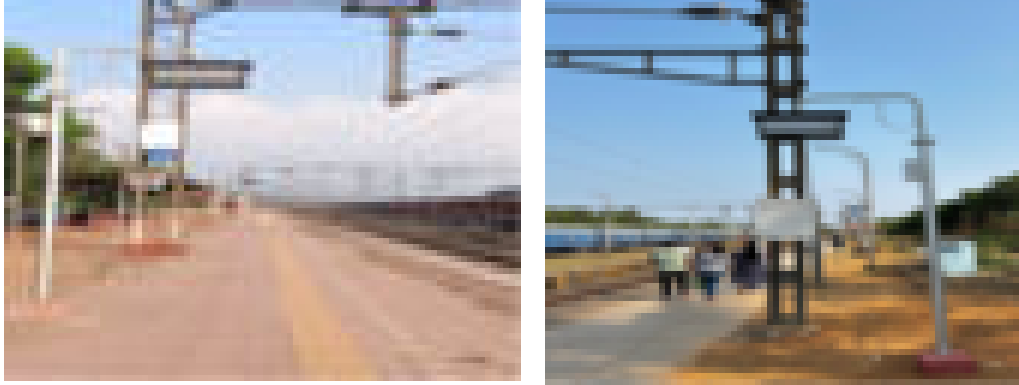
(Coach Guidance Display Boards installed on platform no. 1 at Chiplun & Sawantwadi Road stations)
