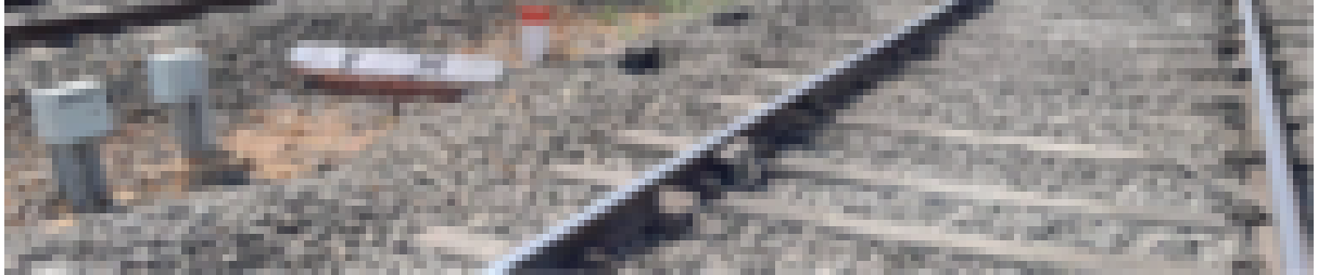
(Dual Detection Point of MSDAC installed at Achirne Station Yard)
